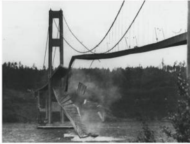
FIGURE 13.26 Collapse of the Tacoma Narrows Bridge—only four months after its opening in 1940—followed the resonant growth of large-amplitude oscillations.
